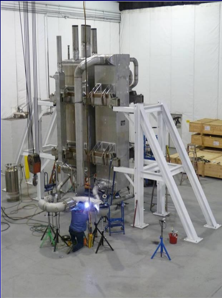
Upper Cold Box Heat Exchangers
