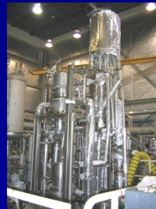
Typical 2K Cold Box Internal Piping
