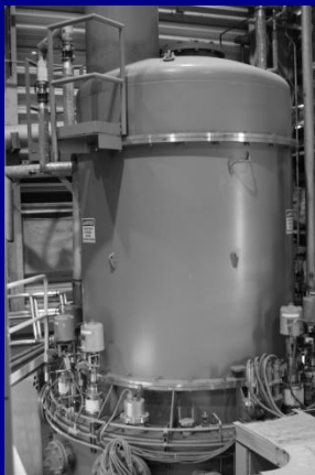
2nd set of Cold Compressor (2K Cold Box) 245 g/s
